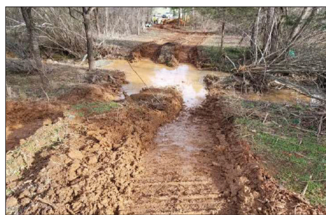
This photo shows stream and streambank damage from an excavator driving through Haven Creek on the property of Mosaic at Chatham Park. The photo was taken during a county inspection on Jan. 9.
