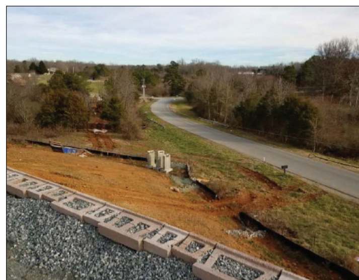
Chatham County Watershed Protection Department inspectors snapped this photo of land disturbance outside approved disturbance limits at Mosaic at Chatham Park during a Jan. 9 inspection.
